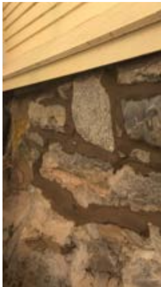
Before and after of the foundation repointing work at the John Paul Jones House
