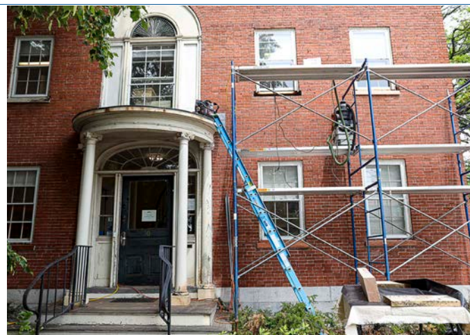
Repair work on the Morton-Benedict facade removed staining on the bricks and made repairs to exterior woodwork.
