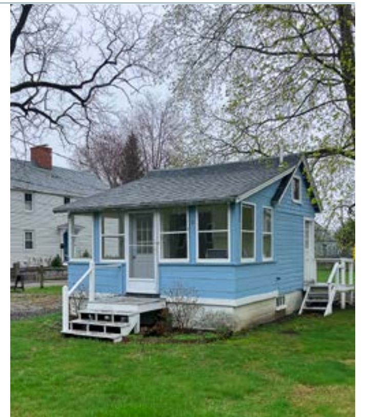
The condition and location of the Candy Cottage at the time of the advocacy alert in April, 2025.
